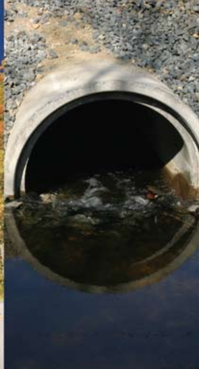
INDUSTRIAL EFFLUENT MONITORING
